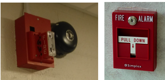
Old fire alarms will be removed and replaced with a new state of the art system incorporating additional pull stations.
