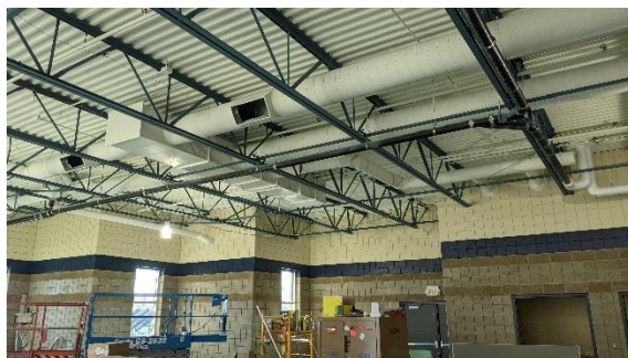
Recent progress on the Weight Room Addition includes installation of exterior glass and painting of the roof deck and structural steel joists.
