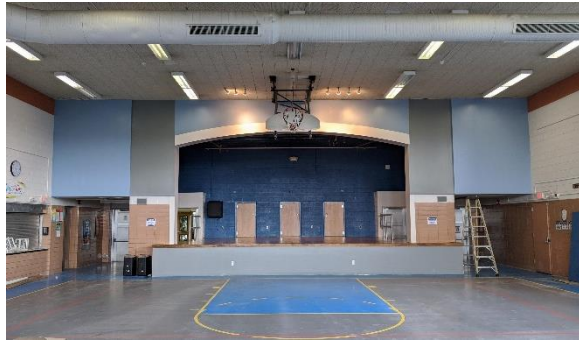
Recently completed work at Schofield Elementary includes new drywall, paint, and stage floor stain.
