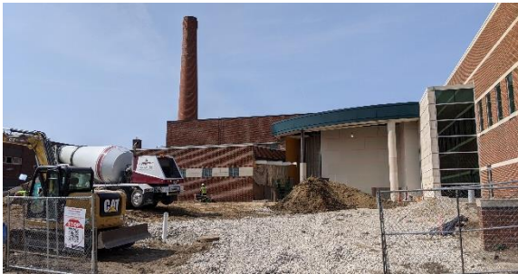
Ground-breaking for the new Fitzgerald High School Weight Room addition began in early September.
